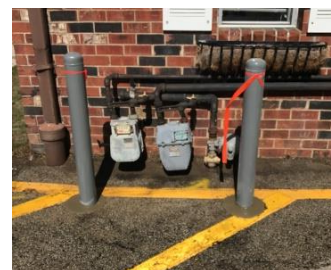
Figure 1- Meter Bollard Provided by Southern Gas Co.
