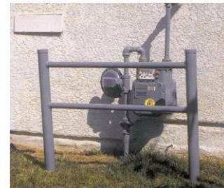
Figure 3 - Guard Rail Provided by Southern Gas Co.
