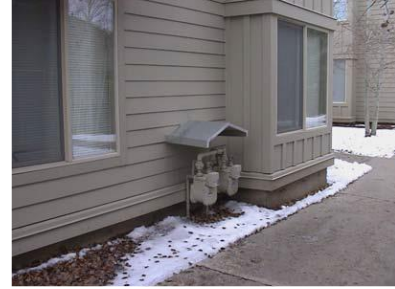
Figure 5 - Gas Meter Enclosure Provided by GTI
